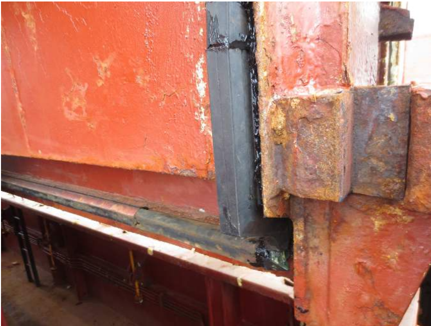
Defective rubber packing.
