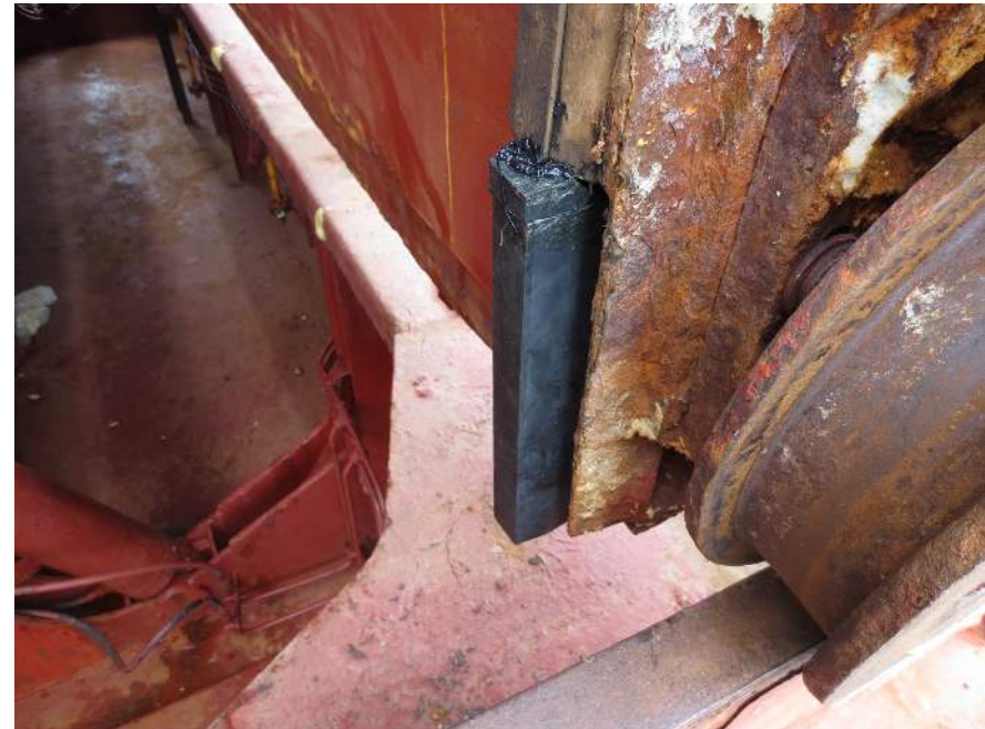
Defective rubber packing.
