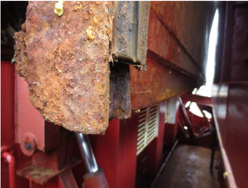
Missing/Poor rubber packing.
